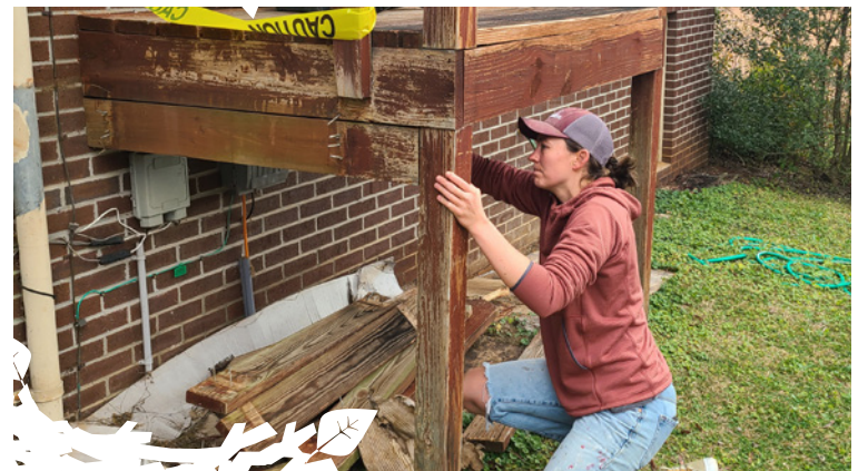
Folks at Home community volunteer power at work, Michelle Thibodeaux replacing our steps.
